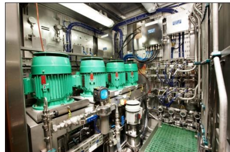
Completed and fully fitted HPU
